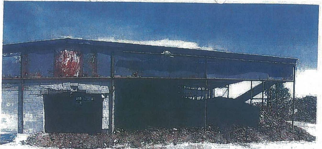
5-13-2010; 11:00 am Photograph # 4 Pecos Valley Meat, Roswell, NM Photographer: Teri Monaghan, NMED/SWB Covered canopy area containing offal and manure piles, facing north.
